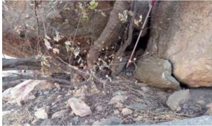
PLATE VII: Collapsed Rock Shelter
